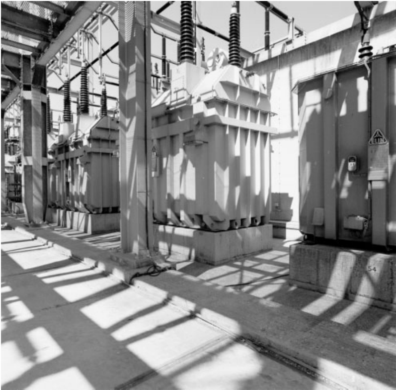
Figure 10.8 Short-circuit transformers. (courtesy of KEMA)
